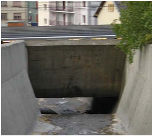
Fig. 1: Bridge designed in model tests to allow pressure flow, in order to increase sediment transport capacity (Modane railway station, Savoie, France)
