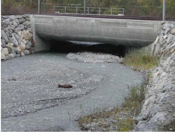
Fig. 5: Bridge with apron allowing pressure flow to cope with high tailwater levels. Crossing of the Simplon railway line over the Gamsa river, near Brig (upstream view)
